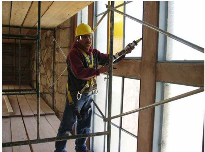
Martin Pizarro caulking gaps in the window frame to keep the cold wind out.
