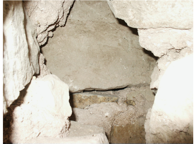
Example of the massive voids in the wall.
